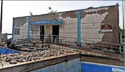
IN DIRE STRAITS: A dilapidated washroom at Kasimedu harbour
